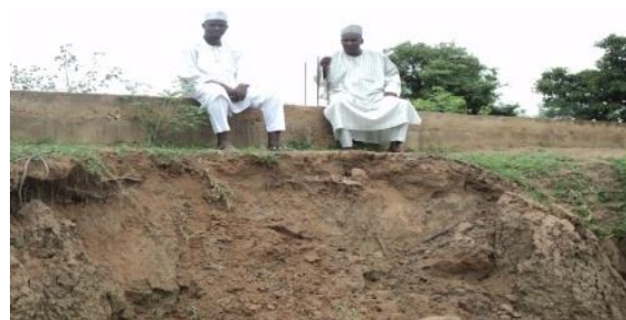
Figure 2h: Gully erosion site at Damare
