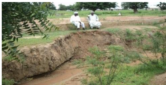
Figure 2b: Gully erosion site at Jabbi-lamba, Girei
